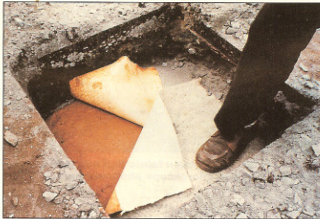
Figure 10: Exhuming needle-punched nonwoven fabric encountered an overlap at location 7, but no performance problems.
