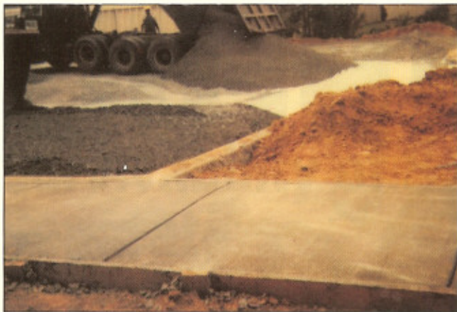
Figure 2: During construction all gravel was placed by dumping unto previously placed gravel.
