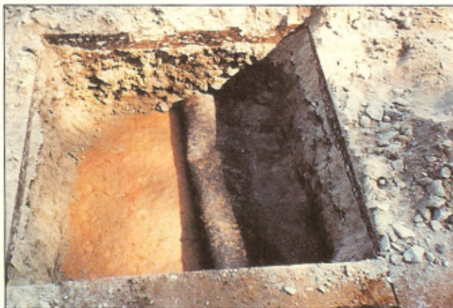
Figure 4: A slit tape woven fabric was exhumed from location 2. Subgrade pumping did not occur, and the fabric showed no signs of damage.
