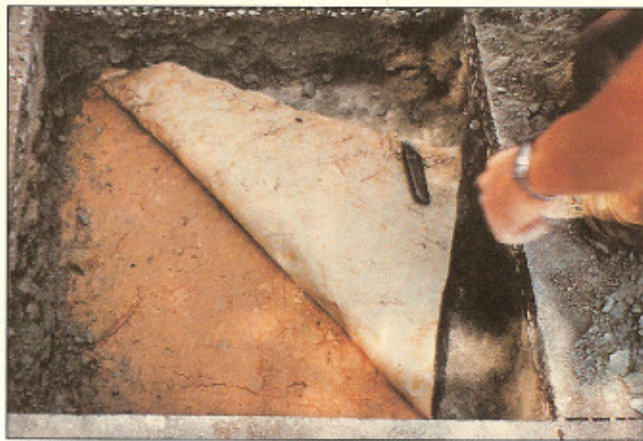
Figure 8: Exhuming spunbonded nonwoven fabric at location 5. Both the fabric and pavement structure were in excellent condition.
