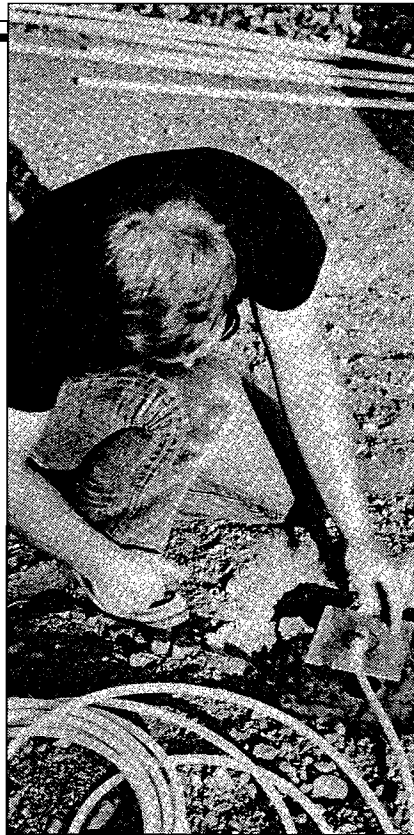
Field instrumentation is designed to measure changes in a single physical property.
